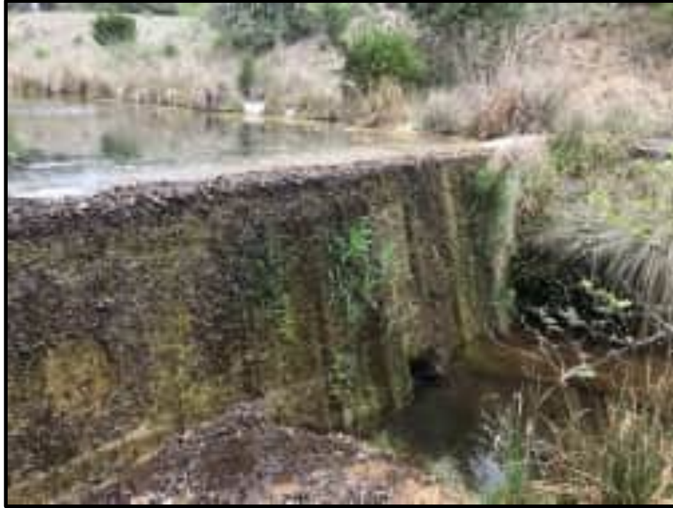
Figure 37. View of Resource 001 showing concrete outlet opening in base of southeast side of dam, looking northeast
